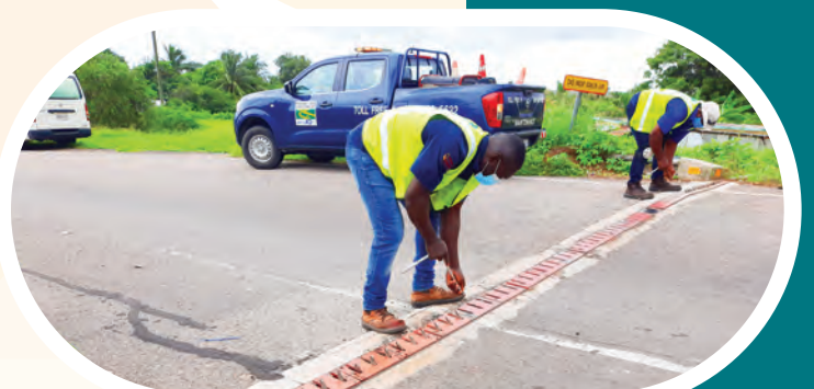
Figure 1.5: Tyre shredders being checked to ensure that they are in proper working order. This has to be done on a bi-annual basis before recertification by the Toll Authority.
