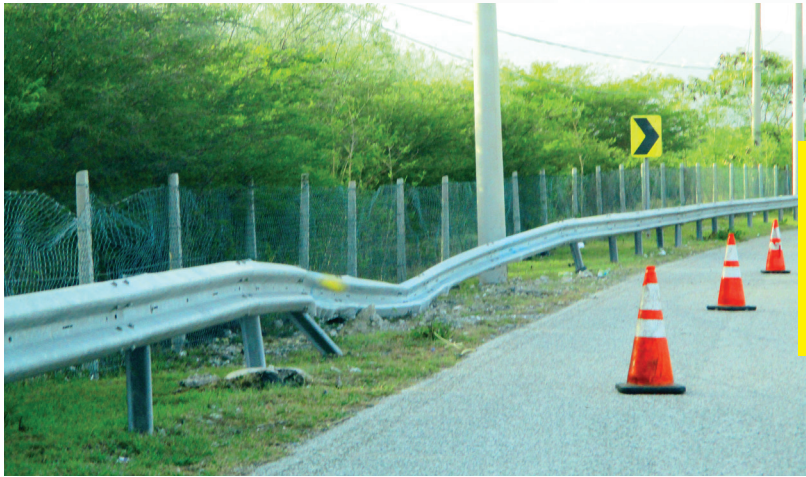
FIGURE 2:1: Shows a damaged guardrail. These traffic control devices serve as a temporary safety measure aimed at alerting motorists of danger.
