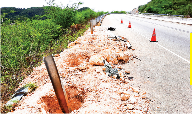
FIGURE 1.4: Shows guardrails being repaired. Repairs to guardrails were scheduled to be completed within three (3) weeks, barring damage due to accidents or related incidents.
