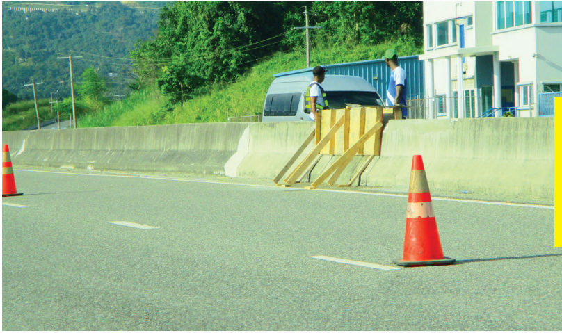
FIGURE 1:7: Shows repairs being done to the Jersey Barrier. These barriers significantly reduce the likelihood of head-on collisions.
