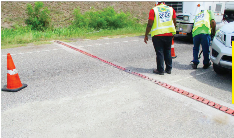
FIGURE 2:2: Shows the removal of concrete that was spilled on the road from a truck.
