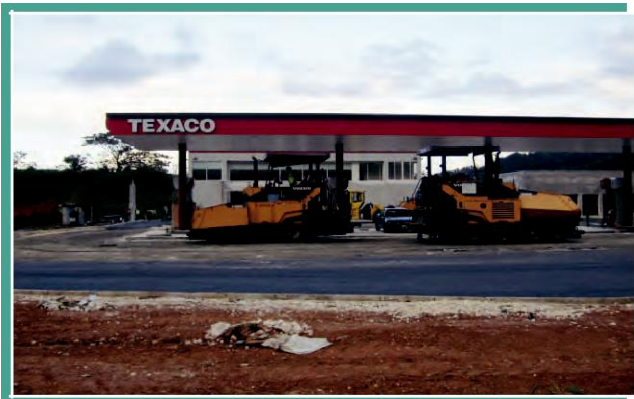
Figure 1.7 – above shows the final touches being done to the new gas station. The gas station began serving customers in 2019.
