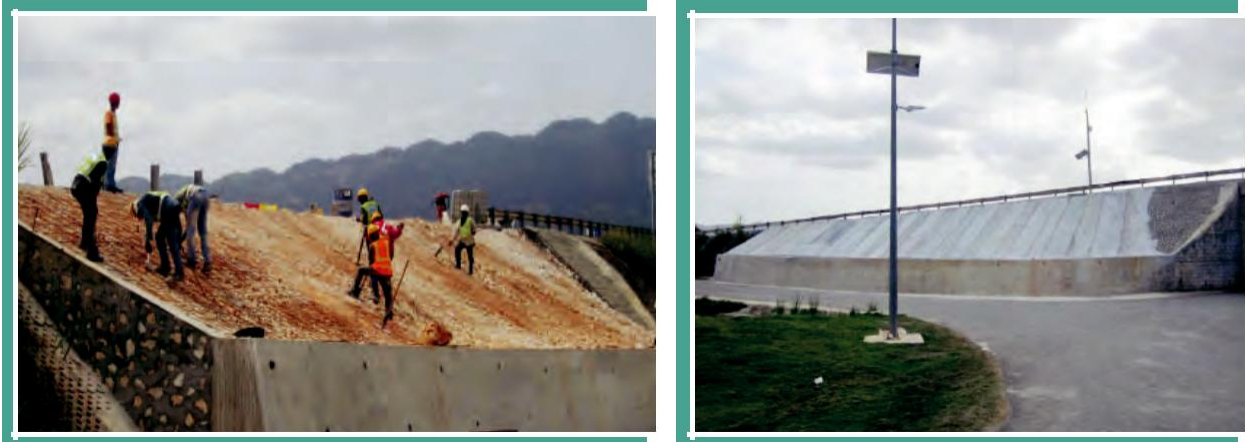
Figure 1.6 - above shows the construction of a retaining wall along the roadway. This was done to prevent the embankment from collapsing.
