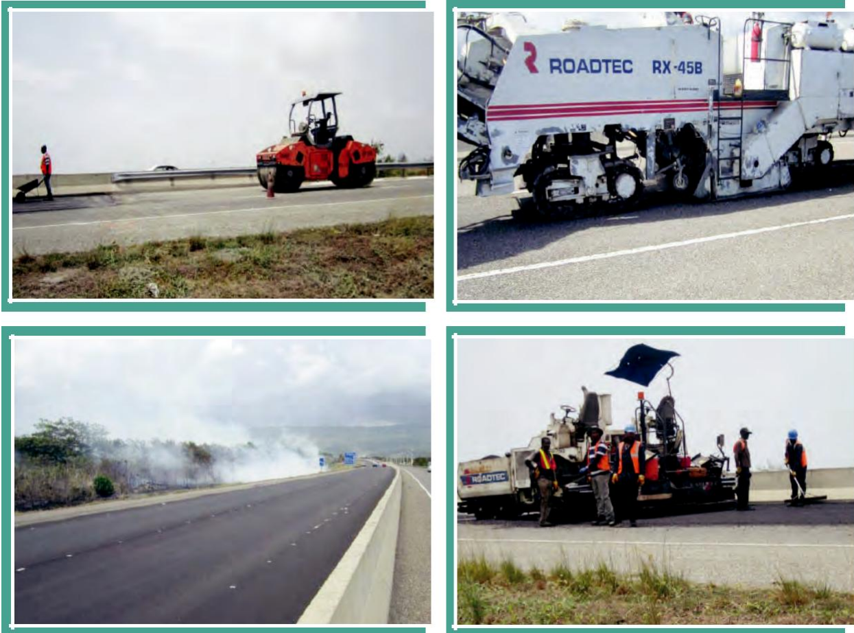
Figure 1.8- above shows images of repairs being conducted on the east and westbound lanes of the East-West Highway. These repairs involved milling to remove the worn upper layer of the existing asphalt, after which a layer of inlay paving was placed on top of the milled surface. Finally, an asphalt overlay was placed on top to finish the process.
