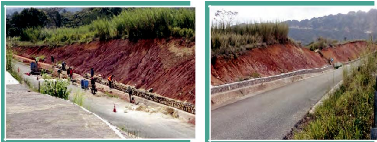
Figure 1.5 - above shows the construction of a rubble retaining wall. This was done to protect the embankment material from being washed down into the V- Drain.
