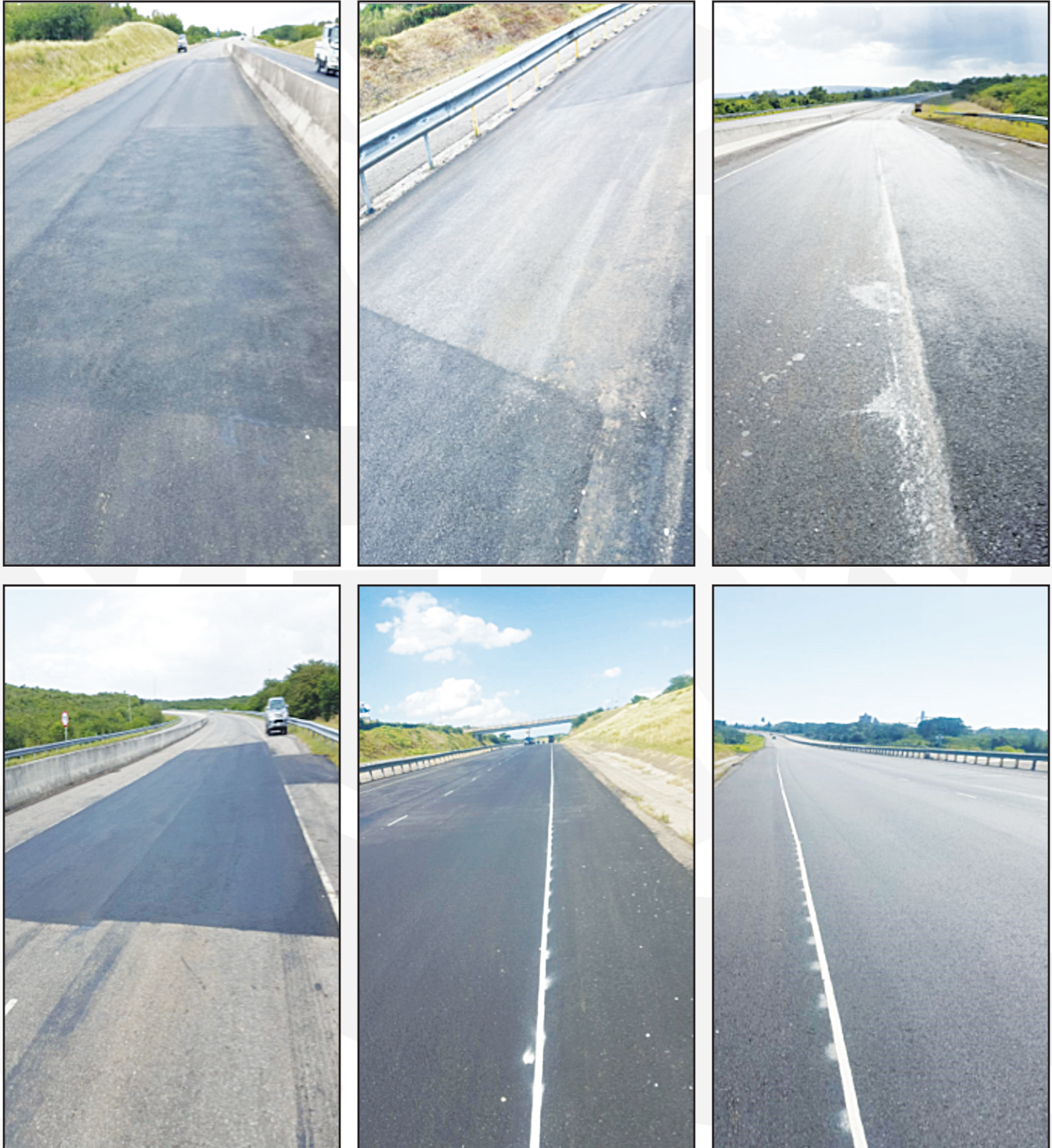
Figure 2.2 Above shows images of micro surfacing repairs that were conducted on the eastbound and westbound lanes of the East-West Highway. Rhinophalt was applied to the road surface to help with water proofing and increase the toughness and aggregate retention on the road.
