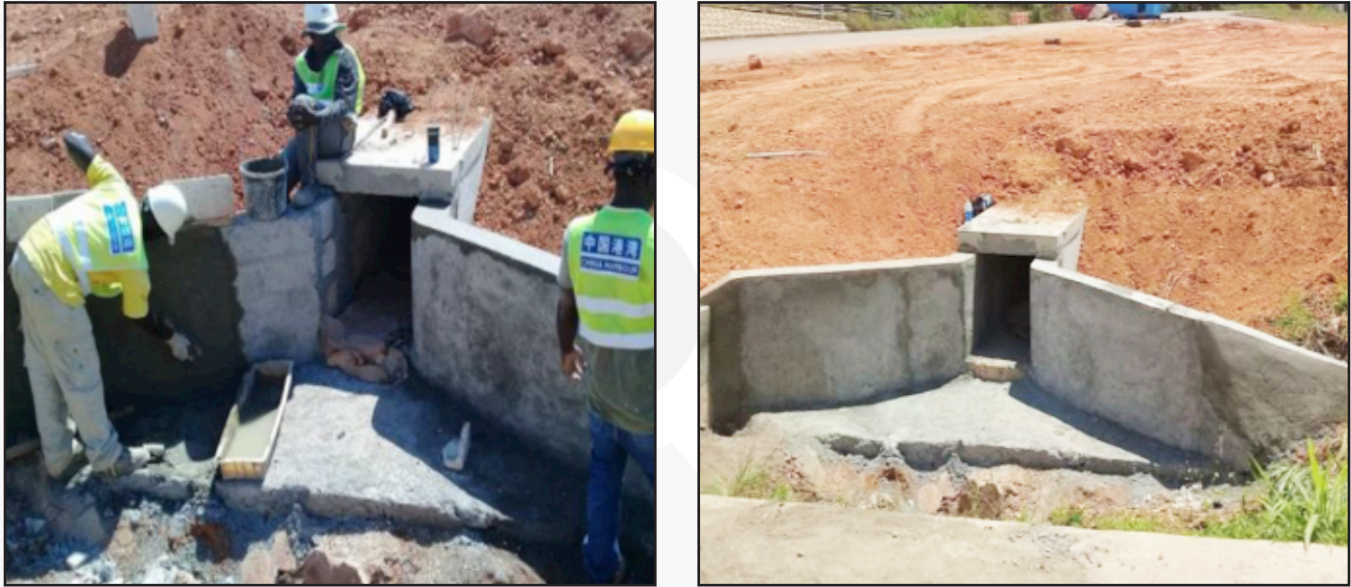
Figure 1.3 Above shows the reconstruction of a drain and the rendering of the wing wall which is located in the vicinity of the Linstead exit of the North-South Highway, as drains along the Toll Roads are crucial in leading water down the slopes to minimise the risk of future land slippages.
