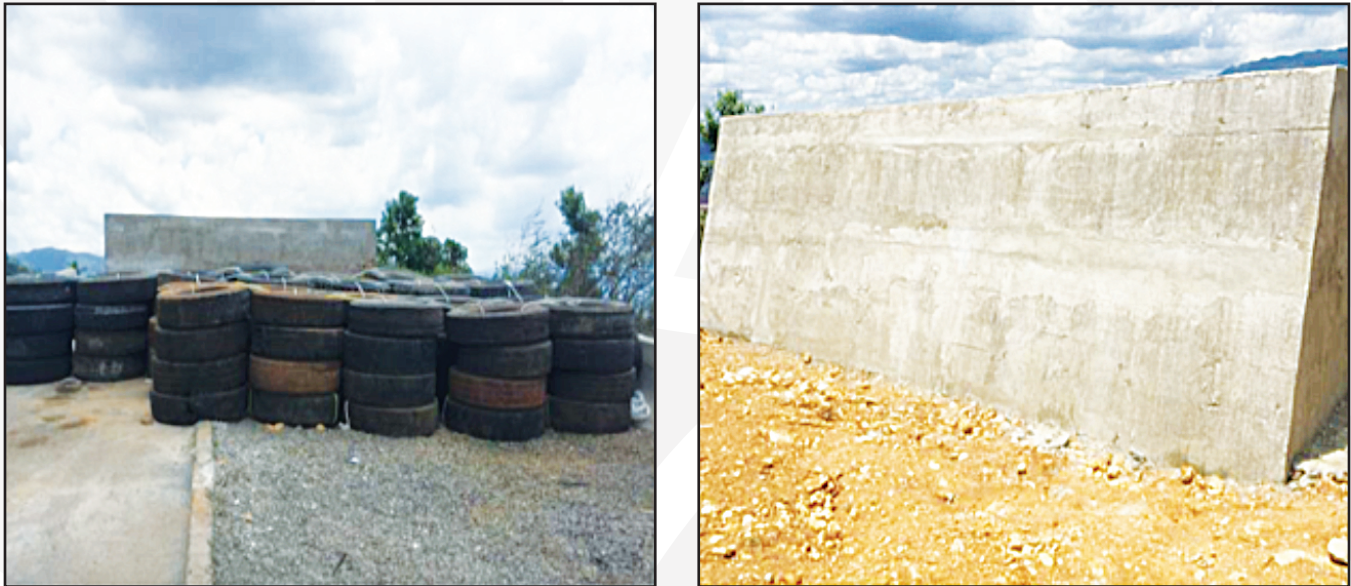
Figure 1.4 Above shows the construction of an energy dissipater wall for an escape lane on the North-South Highway. A lane closure application and a traffic management plan were submitted to the Toll Authority for review and approval as the construction lasted for 72 hours or more.
